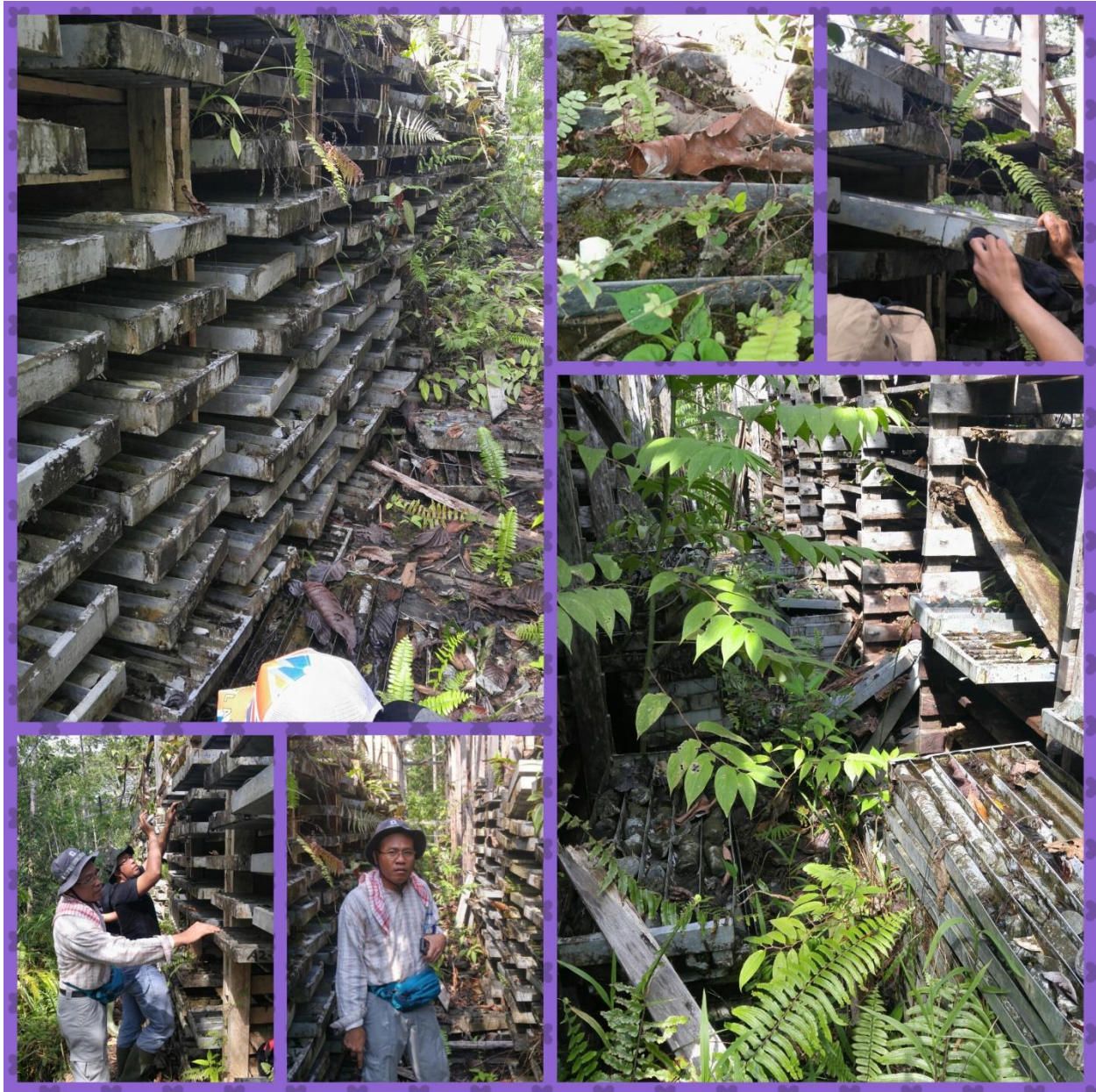
Photo 2. Condition of Tekai Coreshed on 2 November 2016
