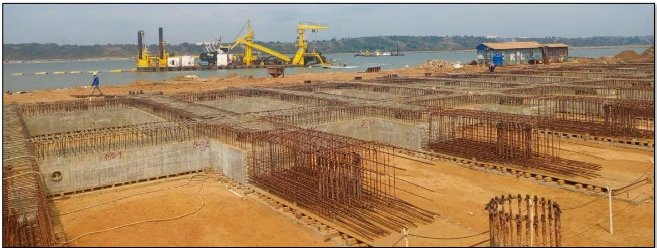
Figure 1 – Progress at the Port of Caio, Cabinda. Expected to be open Q4 2025.
