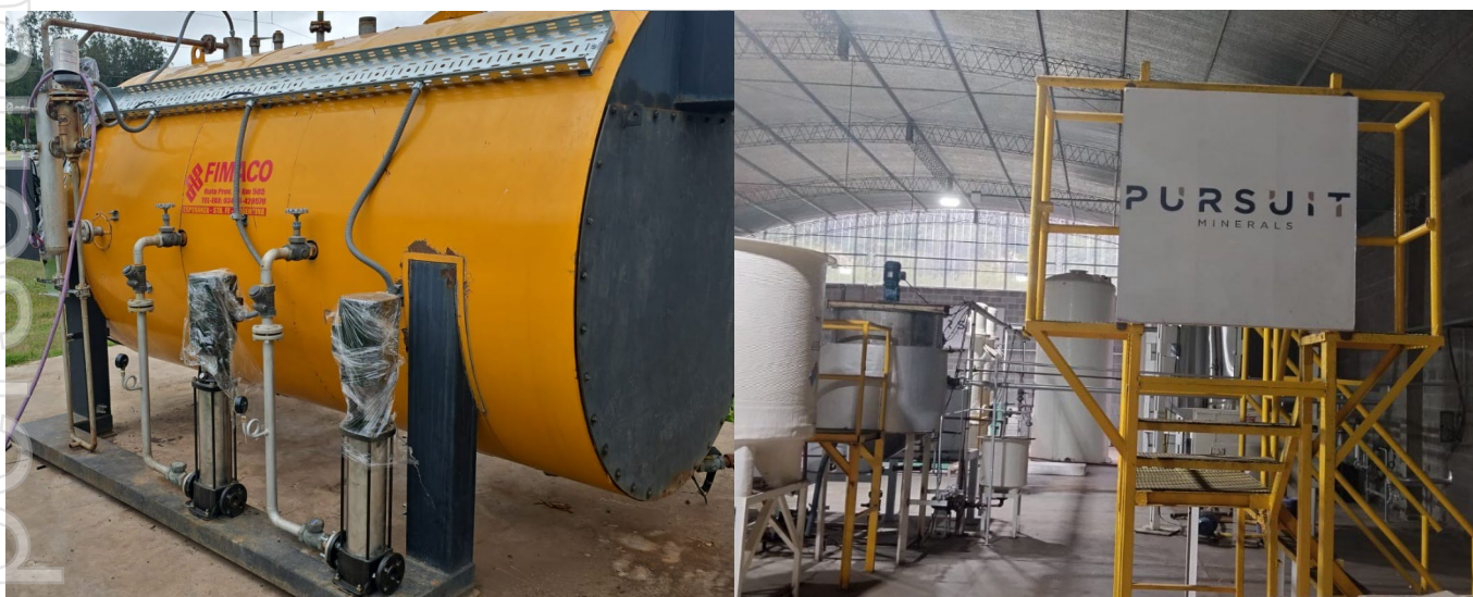
Figure 2 – The boiler installed at the 250tpa Lithium Carbonate Plant in Salta.
