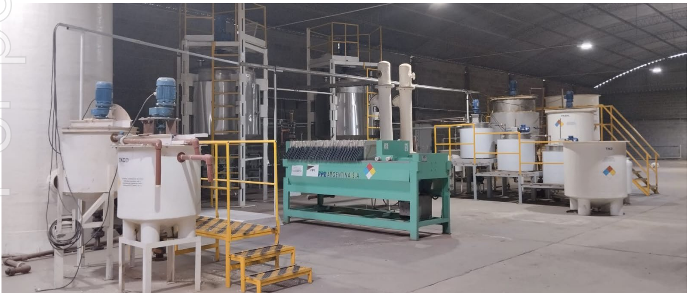
Figure 1 – 250tpa Lithium Carbonate Pilot Plant in Salta, Argentina.
