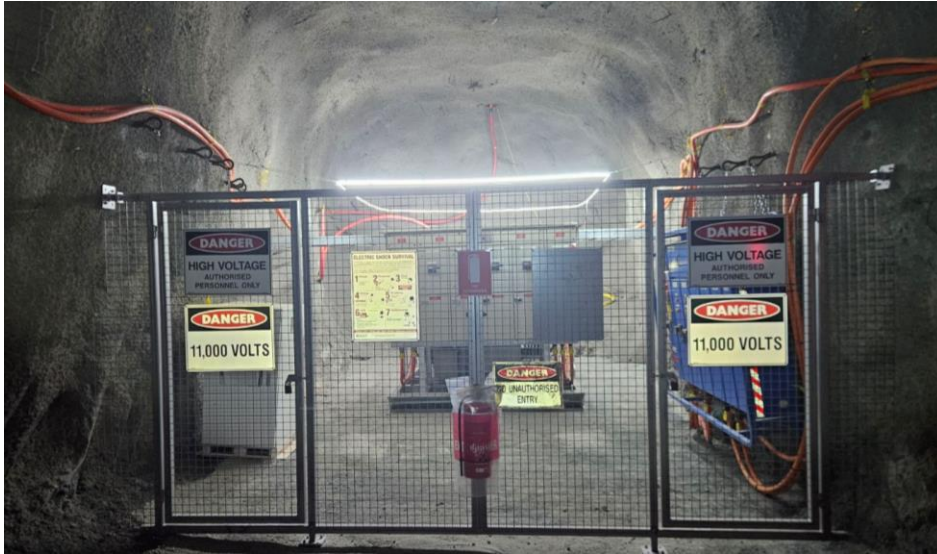
Figure 14 - Underground electrical sub-station
