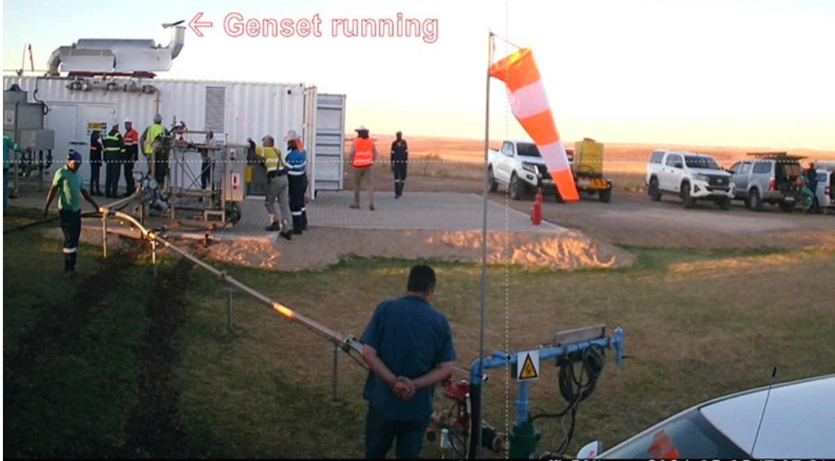
Image above: 1.2mw gas generator powering on KKO gas flow from one pilot production well
