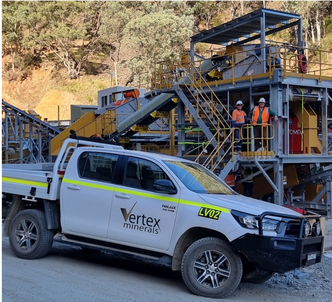
Figure 6 Vertex Directors Declan Franzmann and Roger Jackson keenly on hand at the newly erected ore sorting circuit
