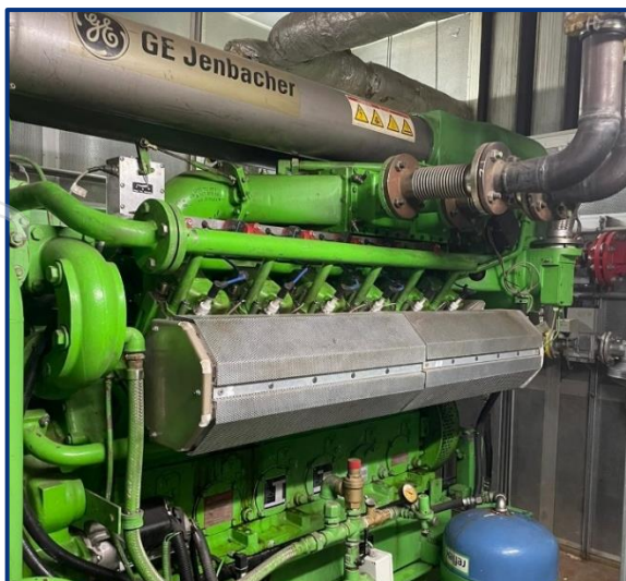
Typical small scale gas fired generator
