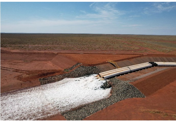
Figure 3: Commissioning of transfer station 2/3
