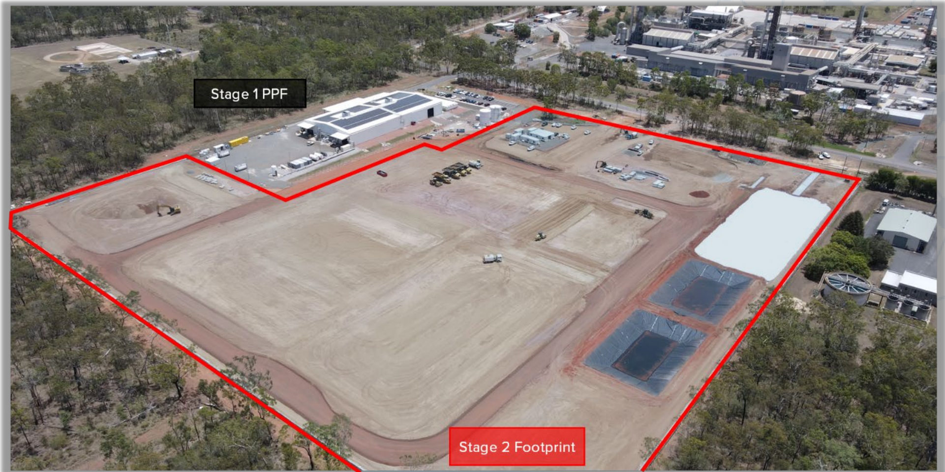
HPA First Project site looking southwest, showing earthworks near completion. Orica Yarwun to the top right of picture.
