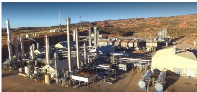
Figure 4: "5 1/2 Nines" Advanced Lisbon Valley Gas Processing Plant.
