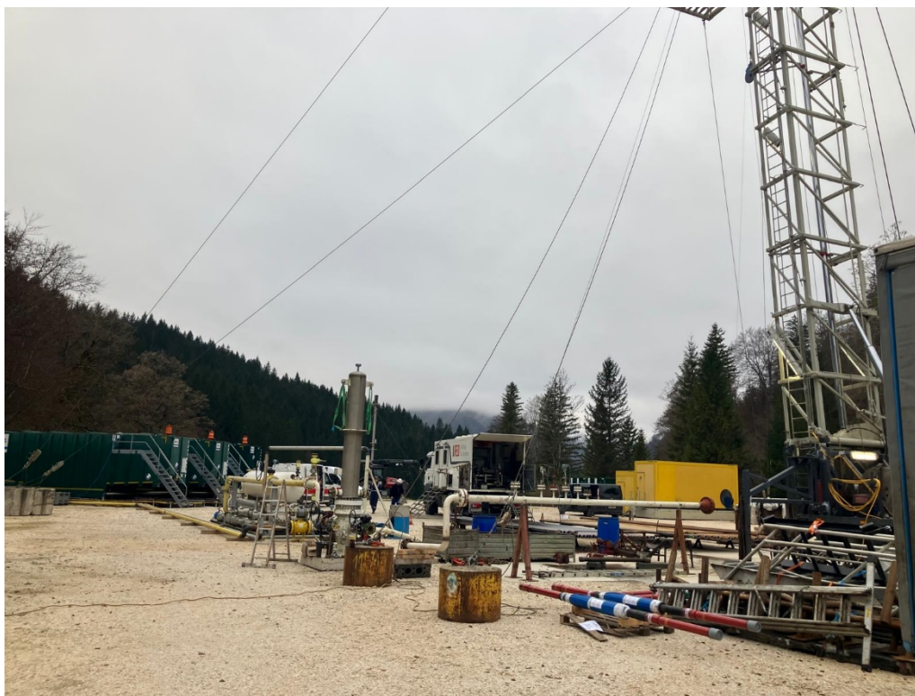
Well completion work and Flow Testing Facilities set up at the Welchau-1 well location for flow testing the well
