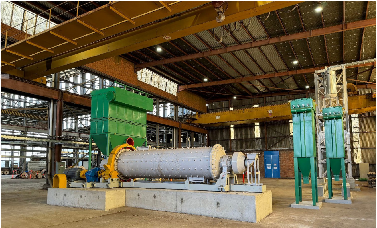
Figure: Briquette civil work completed with major equipment set in position on foundations
