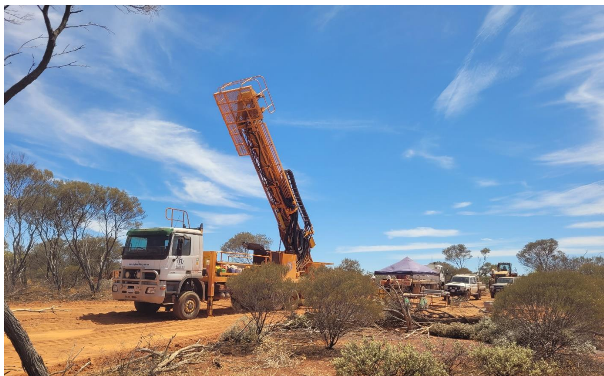
Figure 1: Line Hydrogen Pty Ltd contracted diamond drill rig drilling geotechnical hole for trial open pit as part of heap leach feasibility study
