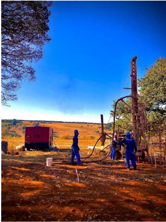
Figure 8: Reverse circulation drill rig in the backdrop of vast pastureland of CODA North.
