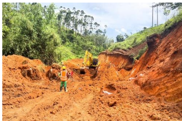
The Tanzanian team commenced upgrading the 3.5km Southern Road leading to the Epanko Graphite Project in the Ulanga District
