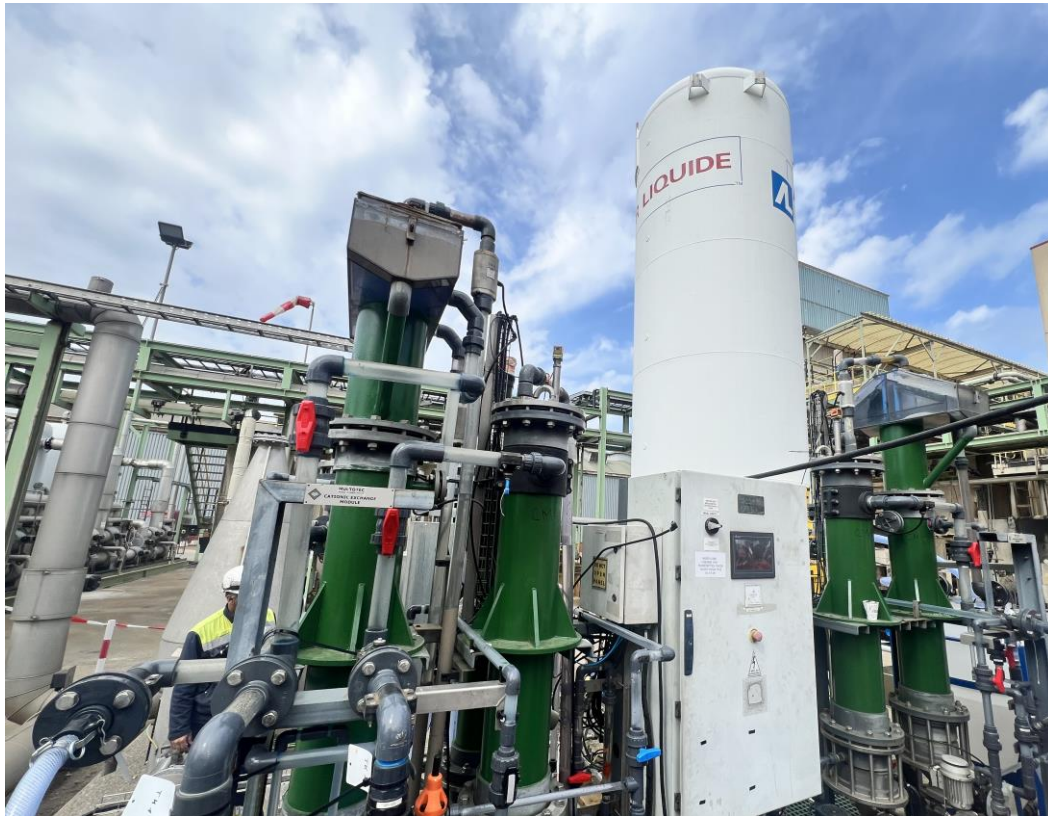
Commissioning of Nyrstar DESALX ® pilot plant
