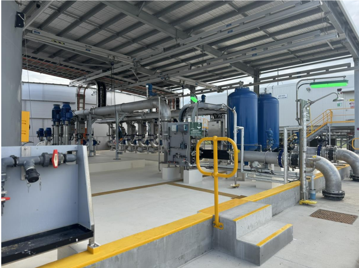
Clean TeQ completed cold commissioning of Townsville Water Recycling Facility in December
