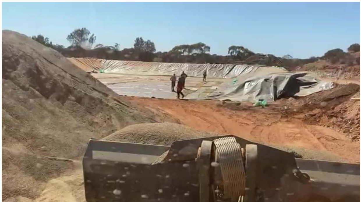
Figure 5: Crushed material about to be loaded into the vat leach facility at East Menzies Gold Project, November 2024
