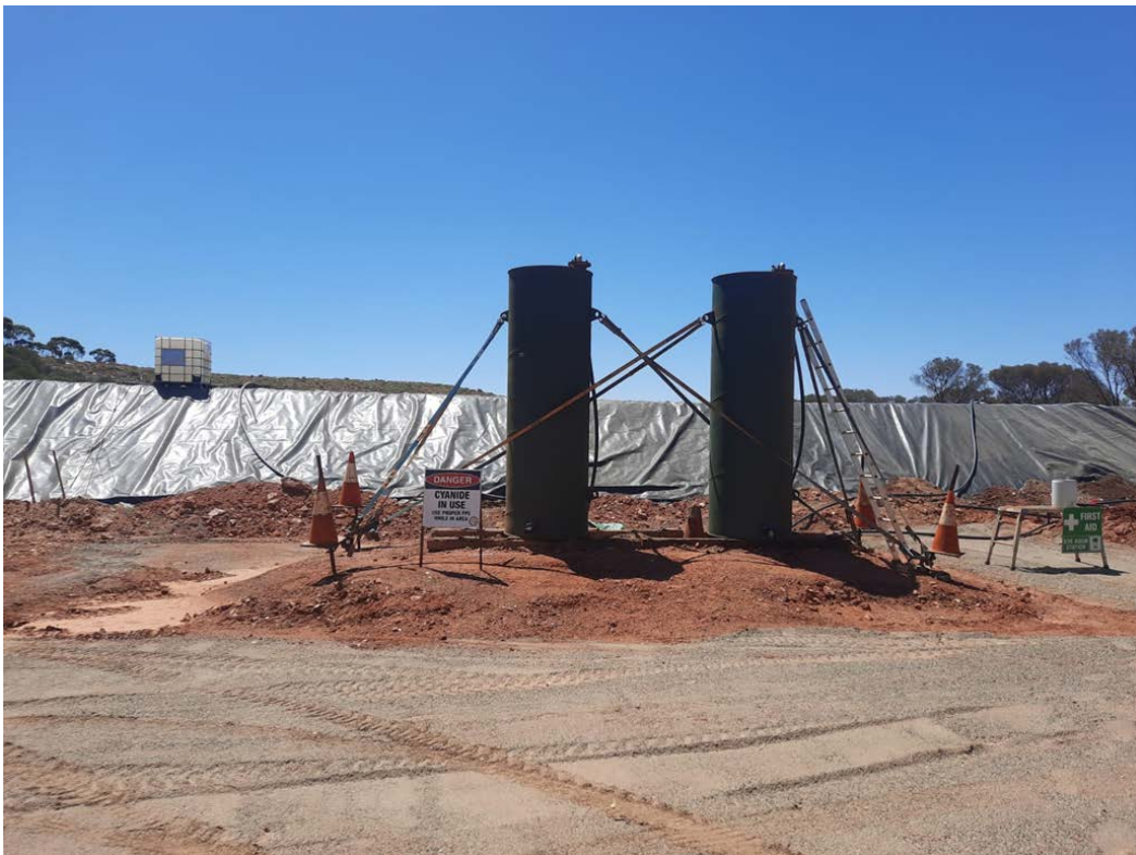
Figure 7: Carbon Tanks in situ at East Menzies extracting and holding onto precious metals, December 2024
