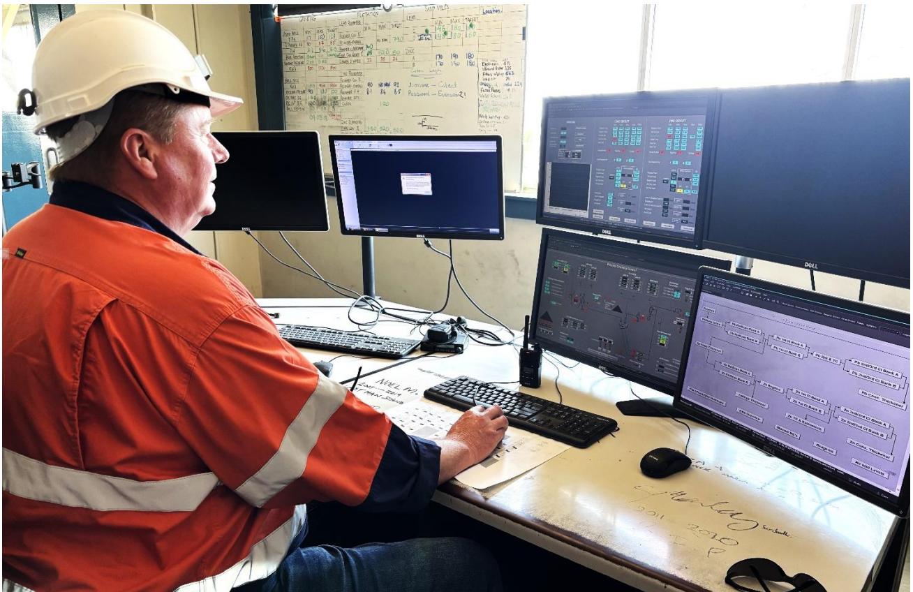
Figure 4: Process plant control and analysis systems upgrade.
