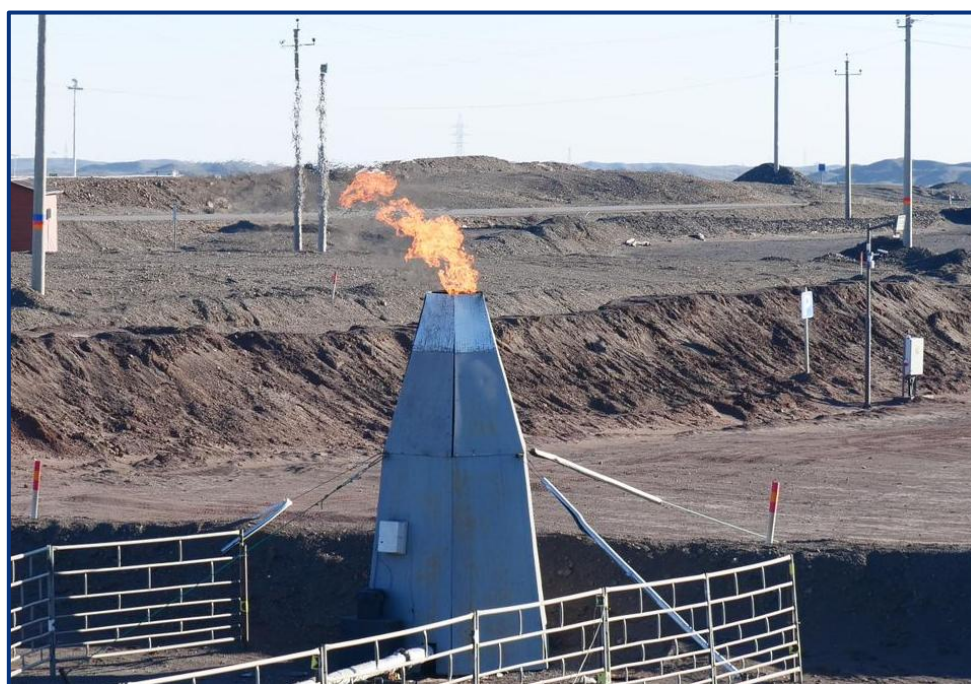
Figure 1: LF-02 gas flare with adjacent local electricity infrastructure
