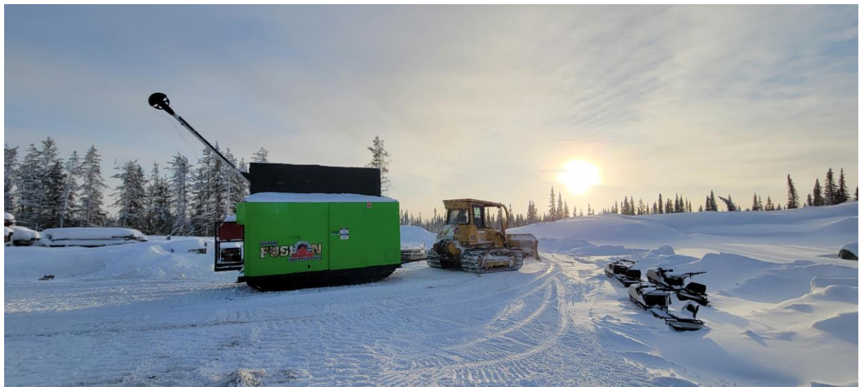
Figure 2: Mobilizing drill rig at the start of the winter road (western end of the CV5 Pegmatite).
