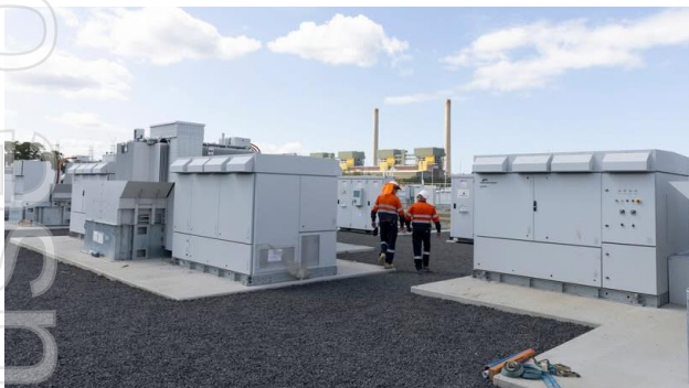
Picture: Eraring battery
