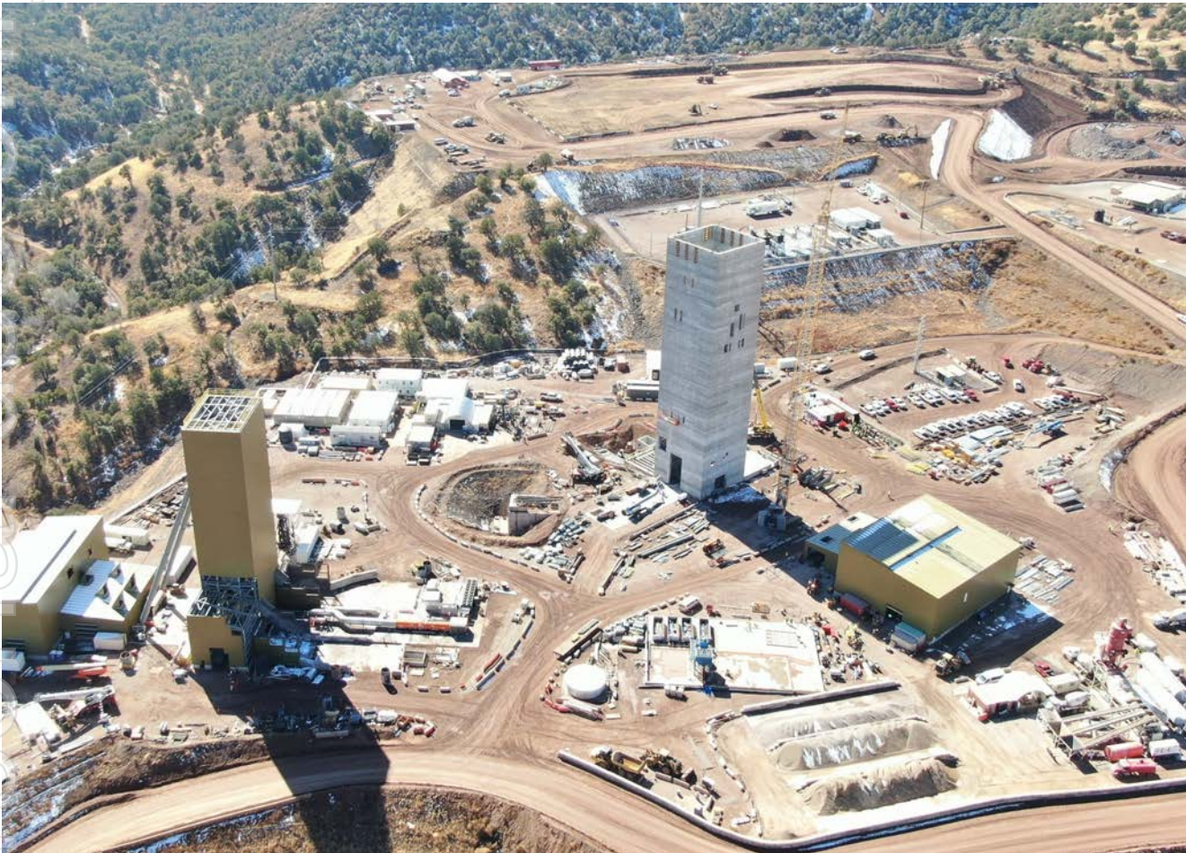
Construction of ventilation shaft (left), main shaft (right) and completed concentrator pad (top)
