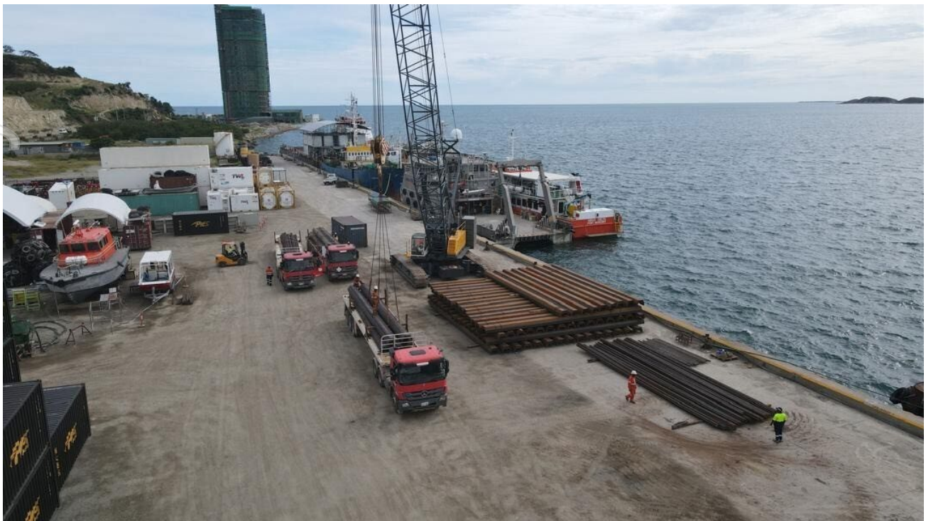
Pictured above: Sheet piling received in Port Moresby before transport to Mayur's CLP
