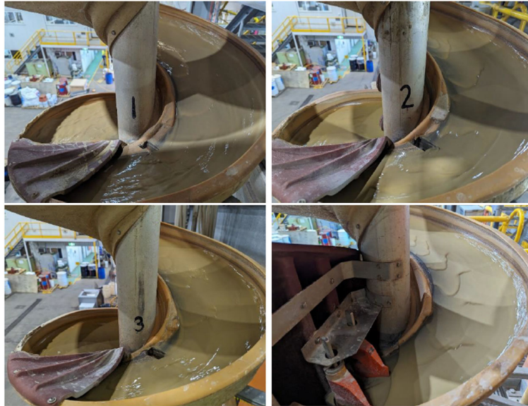
Figure 6 - Wet Concentrator plant, Rougher Spirals
