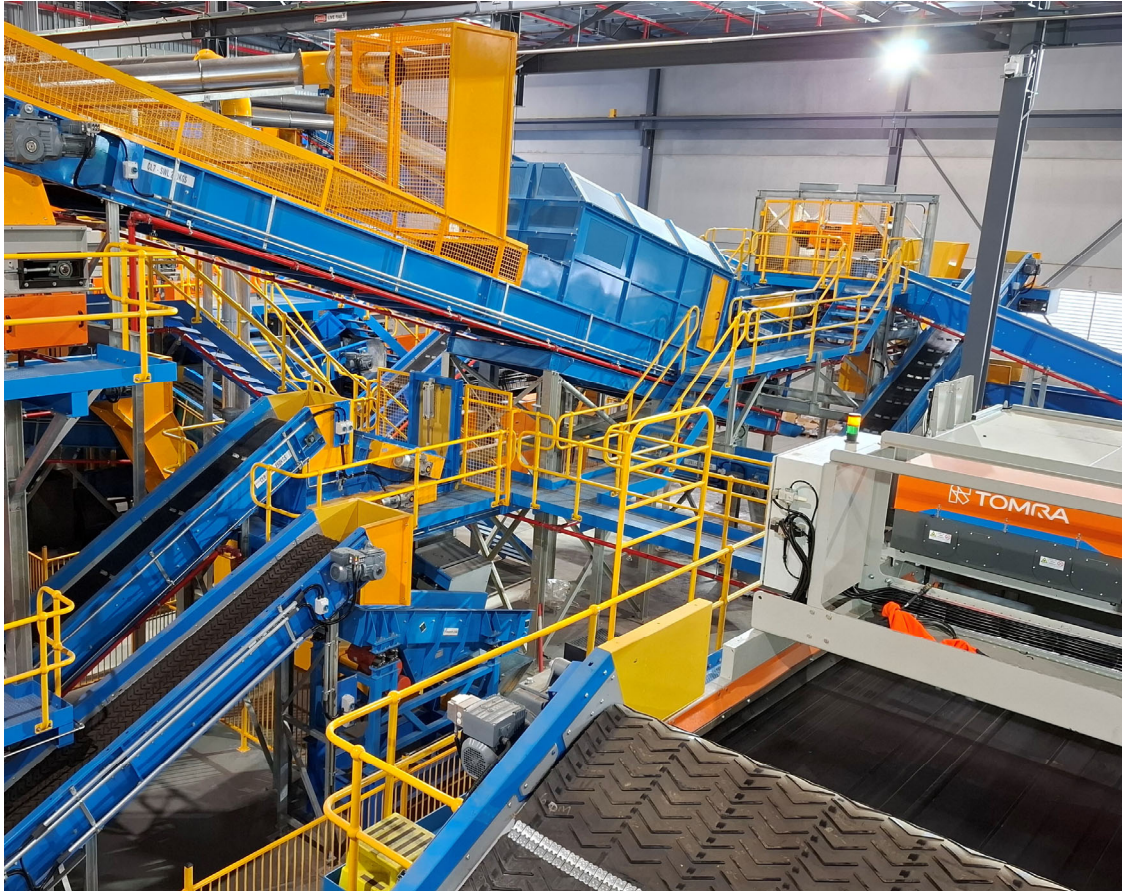
Newly installed Western Sydney Material Recovery Facility processing line in New South Wales
