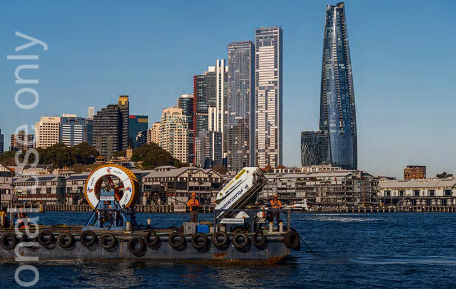
Pictured: Installation of a new fibre optic cable across Sydney Harbour, as part of Telstra InfraCo's InterCity Fibre Network build, NSW
