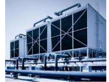
Heating & Cooling Systems
