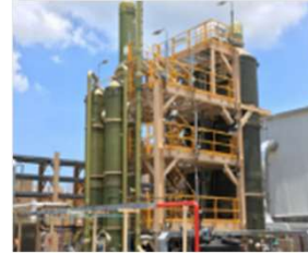
Wet Chemical Scrubber
