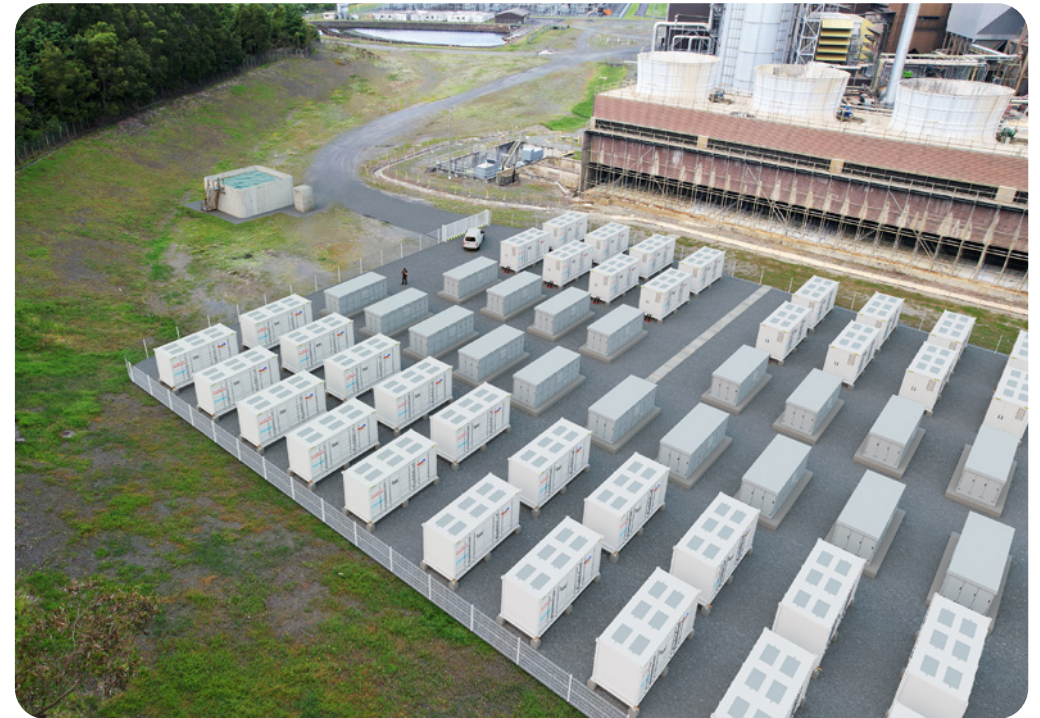
Artist's impression of battery installation at Huntly Power Station
