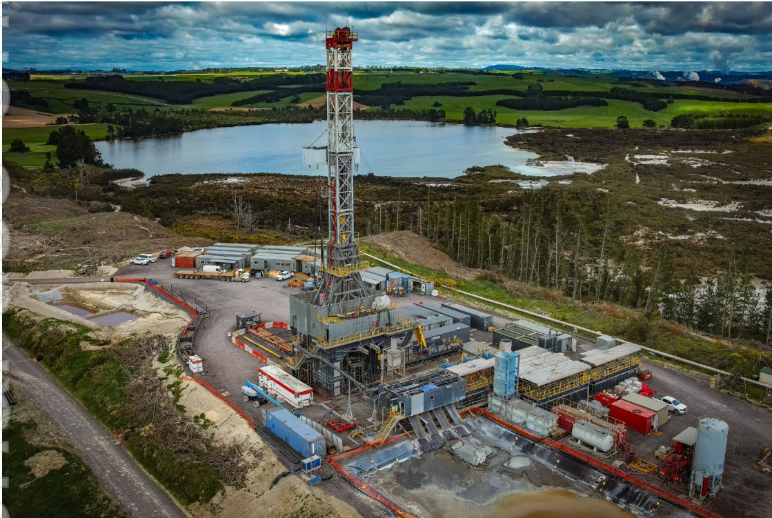
Geothermal drilling rig at Rotokawa
