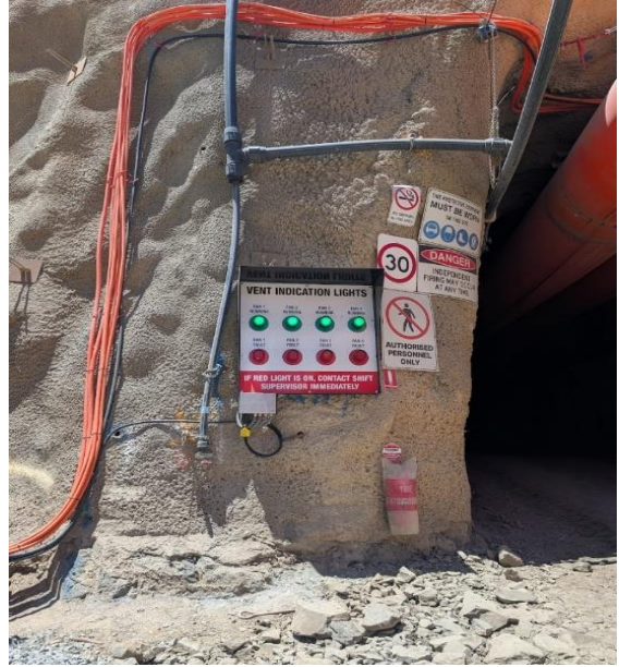
Primary vent fan indicators
