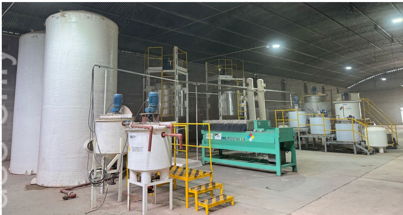
Figure 3 – 250tpa Lithium Carbonate Pilot Plant Ready for Production.
