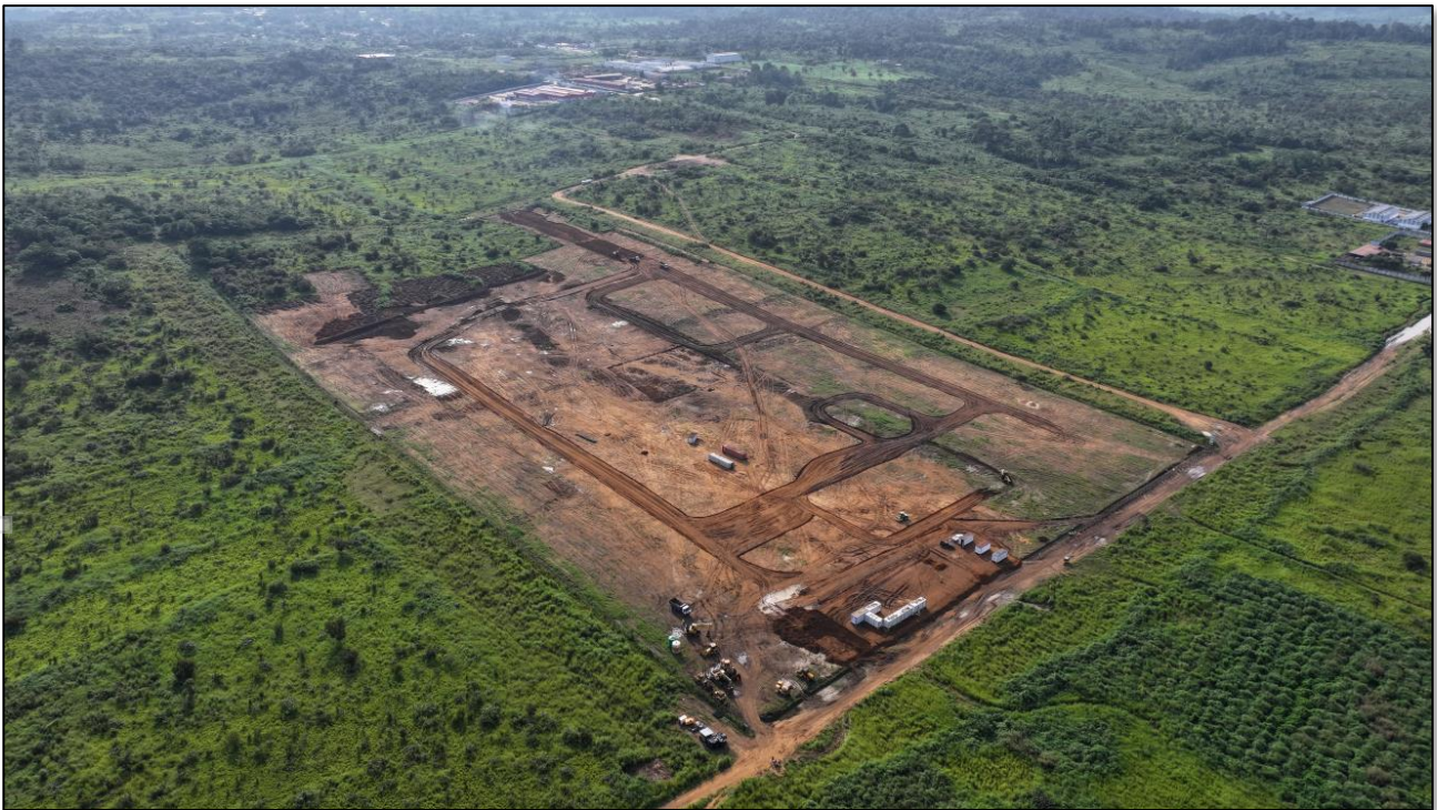
Figure 1 – Site works underway at Subantando, site of the Cabinda Phosphate Fertilizer Plant.
