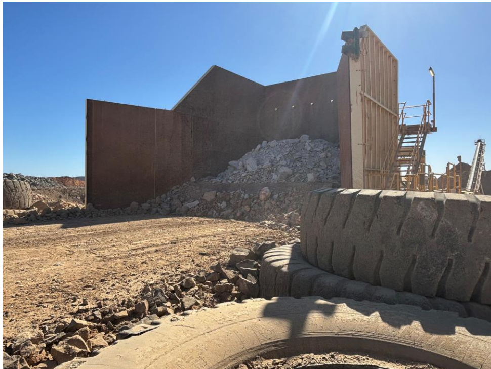
Figure 1 - First bucket of Brightstar ore loaded into the crusher at the Laverton Mill
