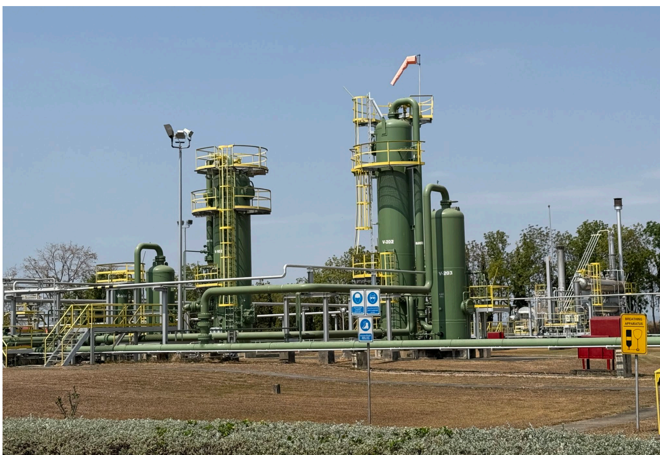
Figure 3 – Nam Phong Gas Processing Plant
