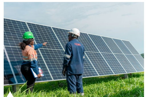
Balama solar and photovoltaic array
