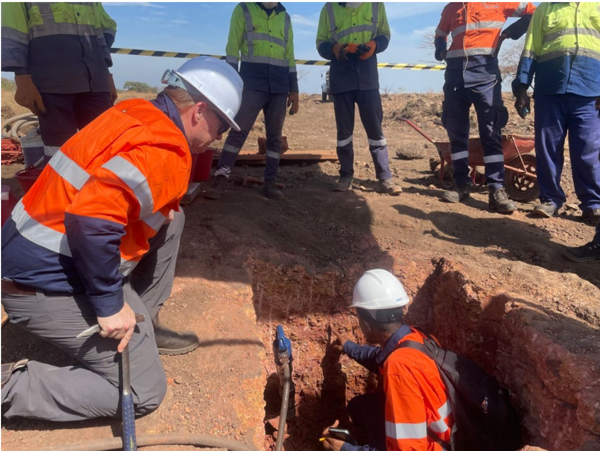
Figure 8. Arrow Bauxite Geologist Mamadou Alieu BAH inspecting bulk sample pit with Arrow's Managing Director
