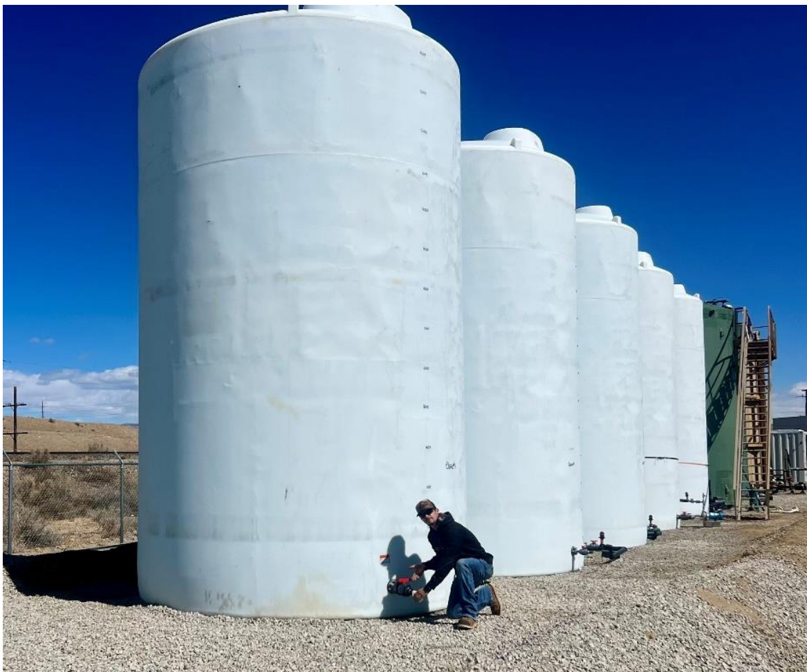
Figure 1: Photo showing the collection and sampling from the near full tanks of lithium chloride eluate produced using KTS DLE at Green River.
