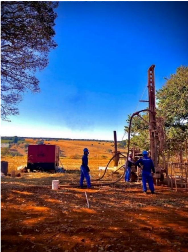
Figure 1: Reverse circulation drill rig in the backdrop of vast pastureland of CODA North.
