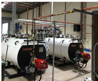
Low Hazard Boilers
