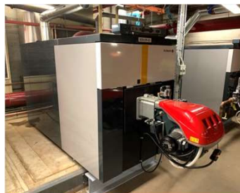
Hot Water Boilers
