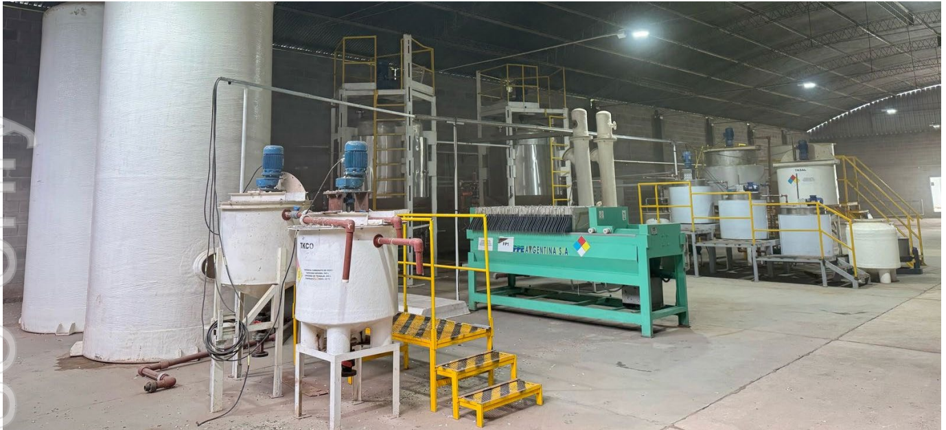
Figure 3 – 250tpa Lithium Carbonate Pilot Plant Ready for Production.
