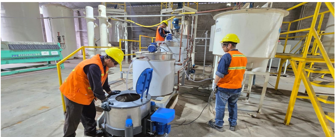
Figure 1 – Pursuit’s 250tpa Pilot Plant producing Lithium Carbonate in Salta, Argentina.
