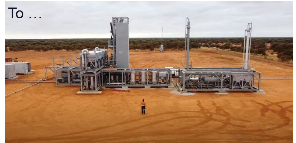
Example of a small-scale LNG Plant in Western Australia
