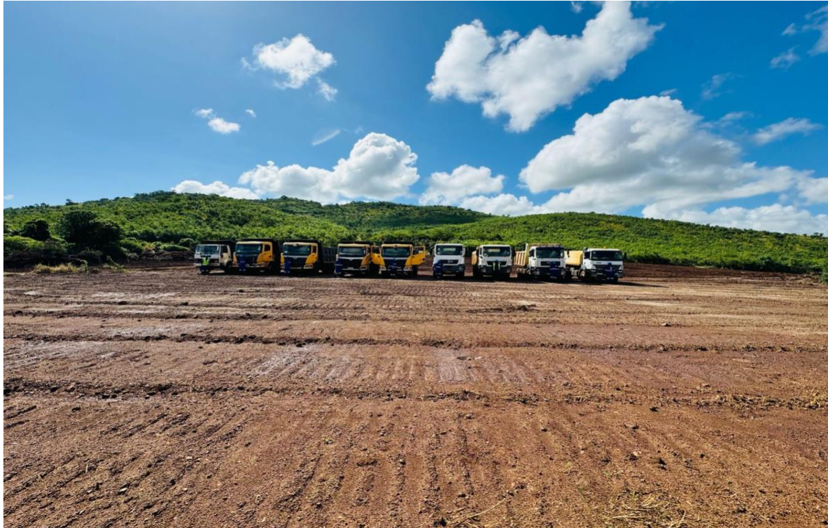
Figure 1 - Mining and Project Equipment laydown area cleared and in use as early works progress across the project footprint.
