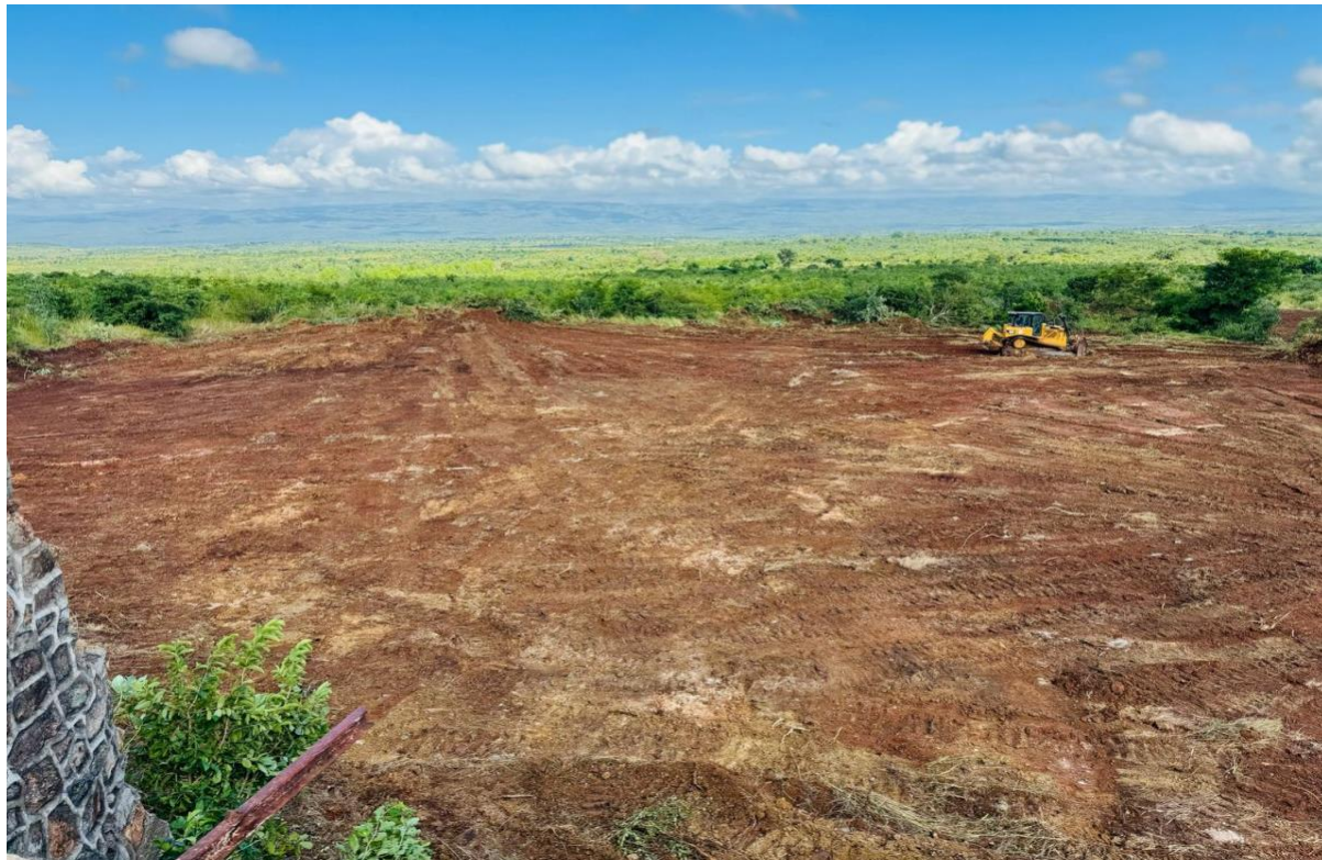
Figure 2 – Area cleared for process plant, product storage, and monazite concentrate loading area.
