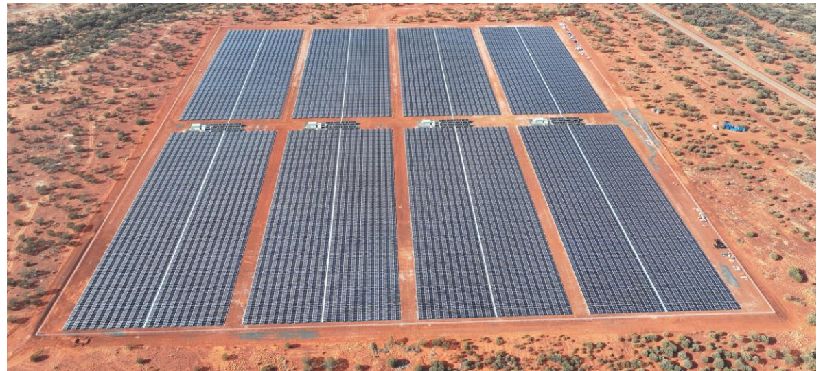
Solar-27MW solar installation commissioned
