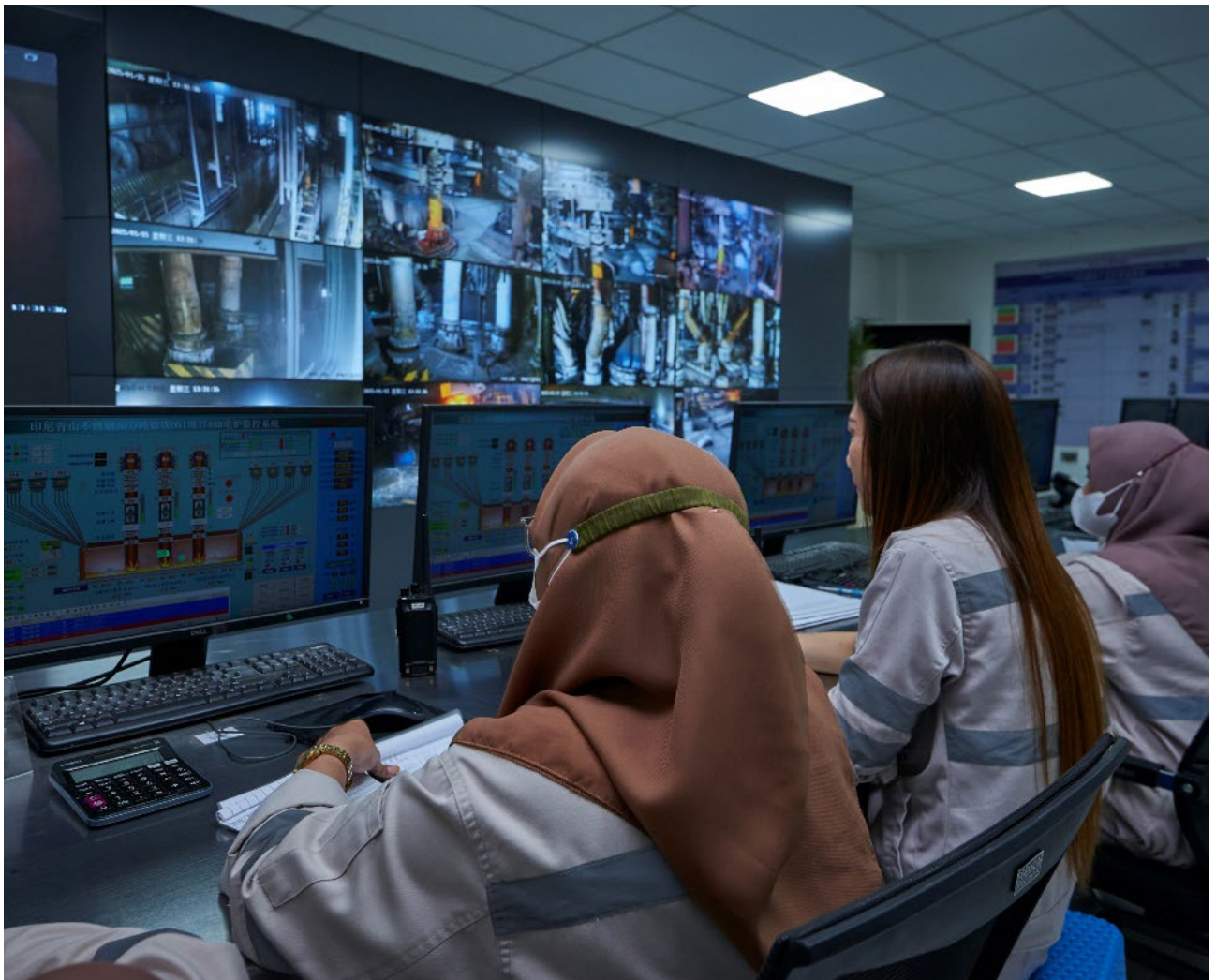
Nickel Industries' RKEF operations control room
