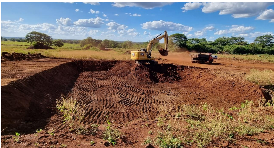
Figure 4. Trial pit excavated by vendor EDEM in May 2023; upper part of alkaline complex is very weathered and suitable for free digging by excavator.
