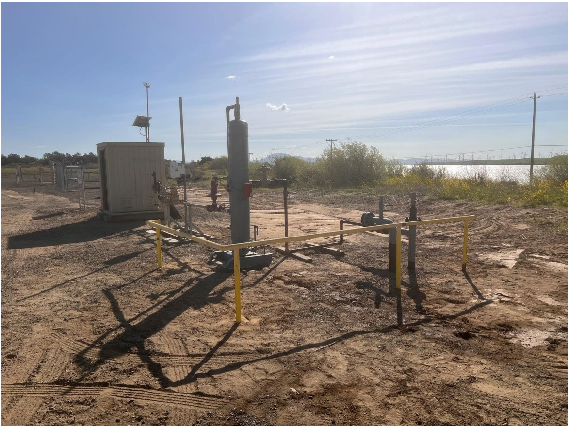
PEOCO Meter (background) with dehydration unit in the Rio Vista Field
