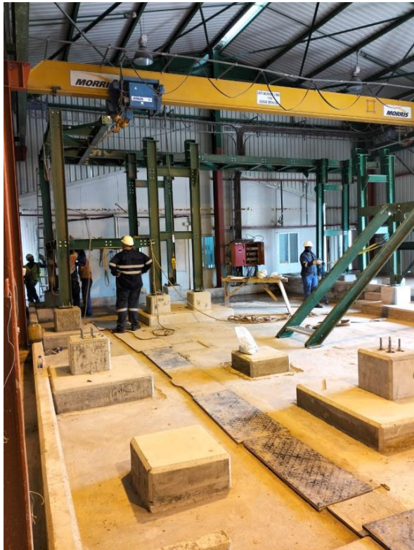
Figure 3: Drying and Packaging – Plinths and foundations ready for structure and calciner installation
