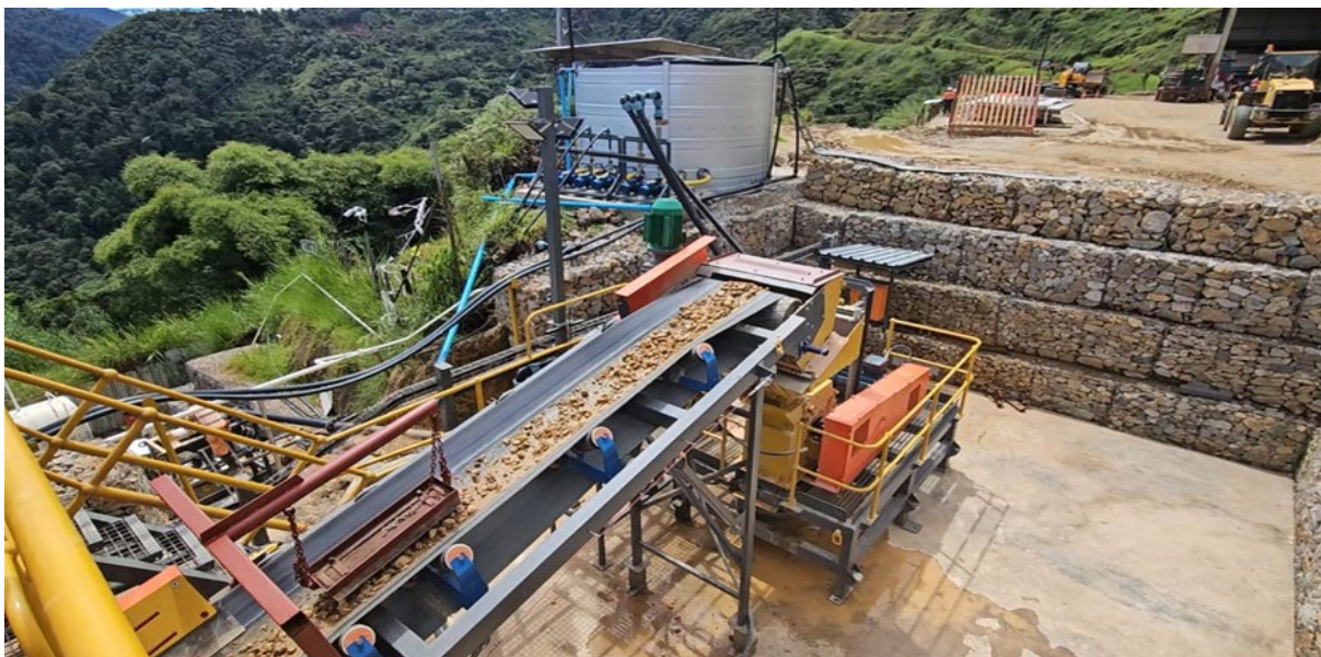
Modular Gravity Plant in operation, February 2025
