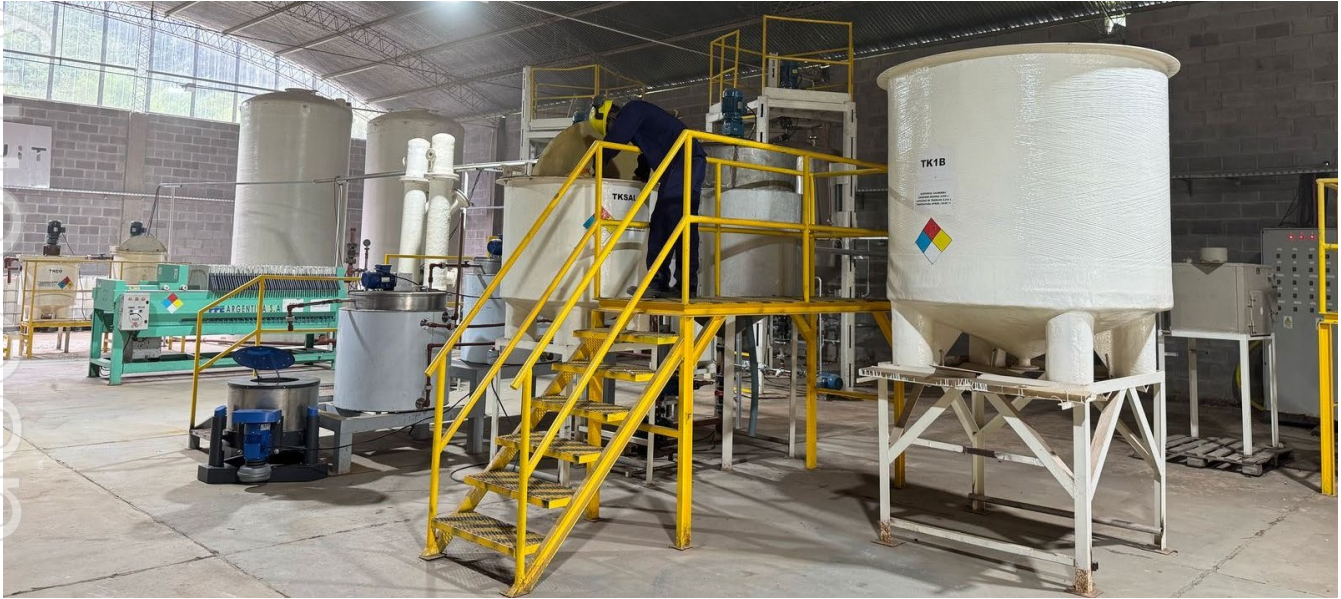
Figure 3: Pursuit's 250tpa Lithium Carbonate Pilot Plant in Salta, Argentina.
