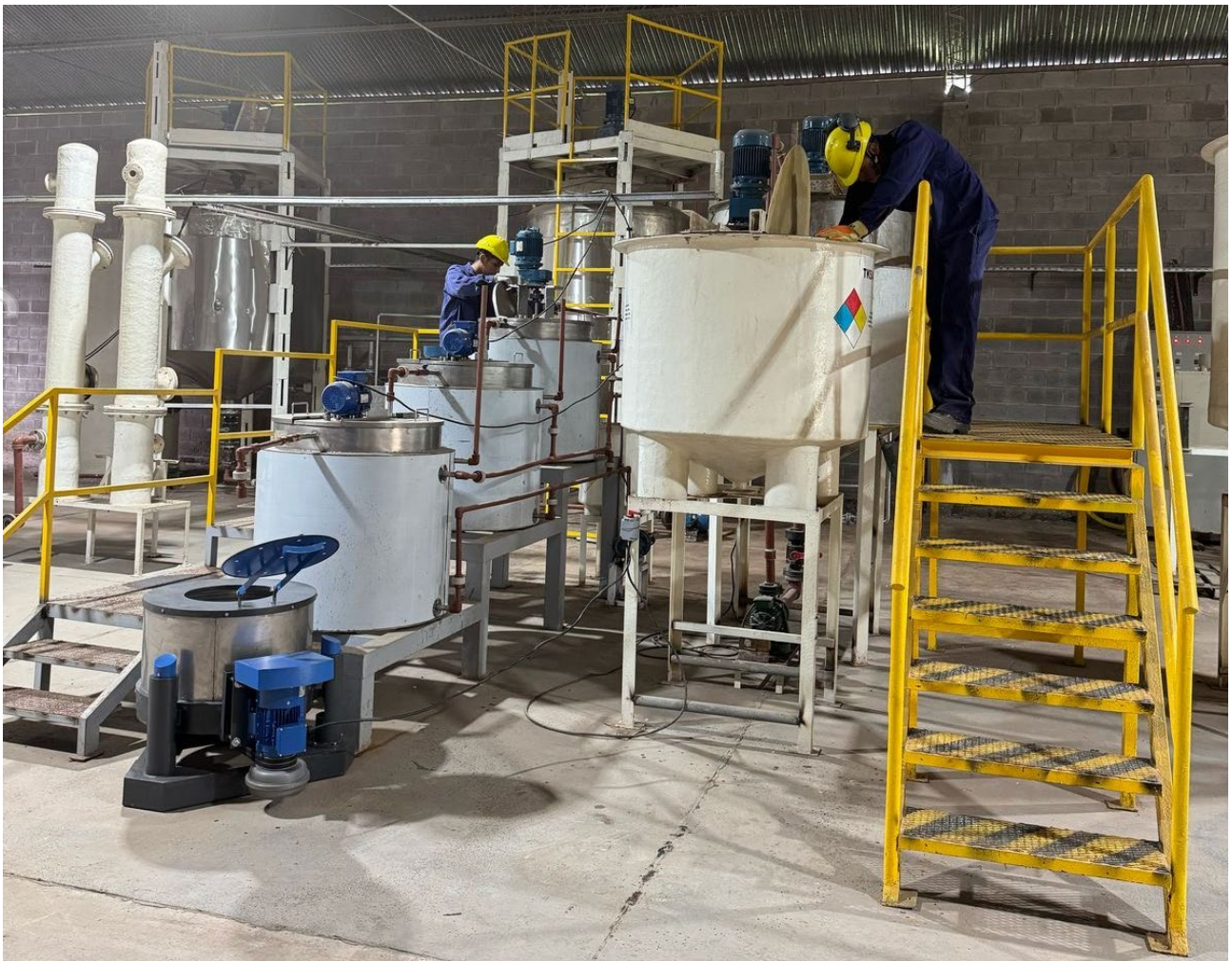
Figure 5: Commissioning in Action: Pursuit Team Conducts Hydrostatic Testing at the Pilot Plant
