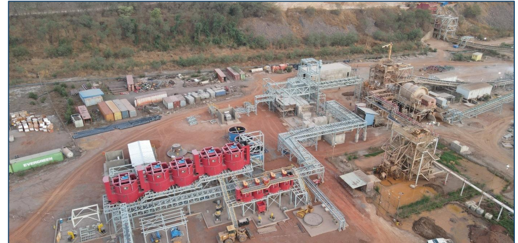
Ball mill and flotation areas under construction. The flotation circuit is now 86% complete, while the ball mill areas is 35% complete
