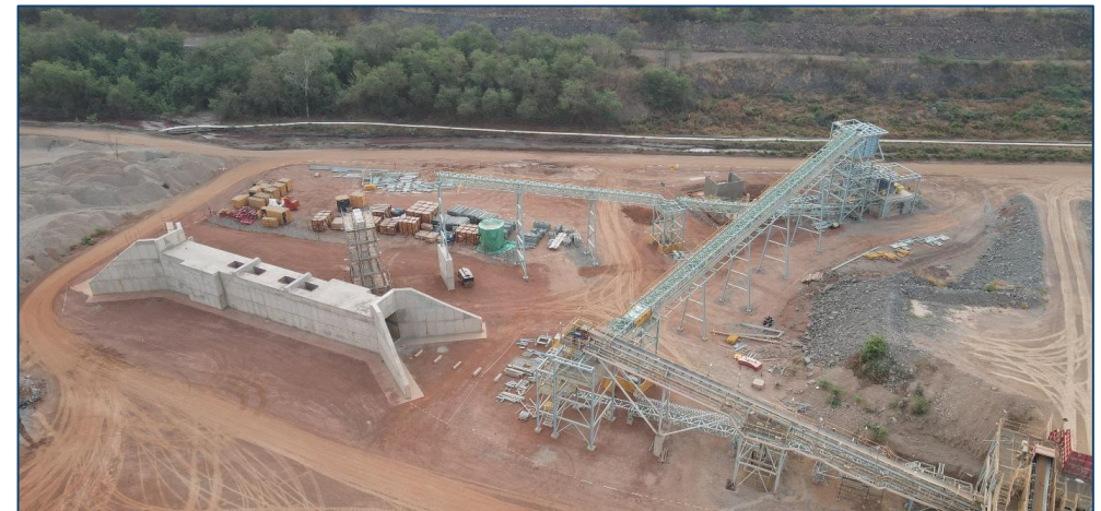
Secondary crusher and sulphide stockpile feed conveyor areas are 50% and 30% complete respectively
